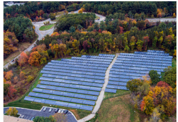
Capital Properties Group | Southborough Solar Field 1,000 kW
